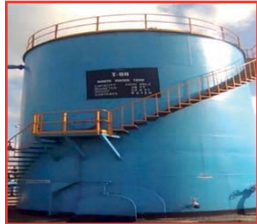
Gambar 62. Oil Storage Tank
